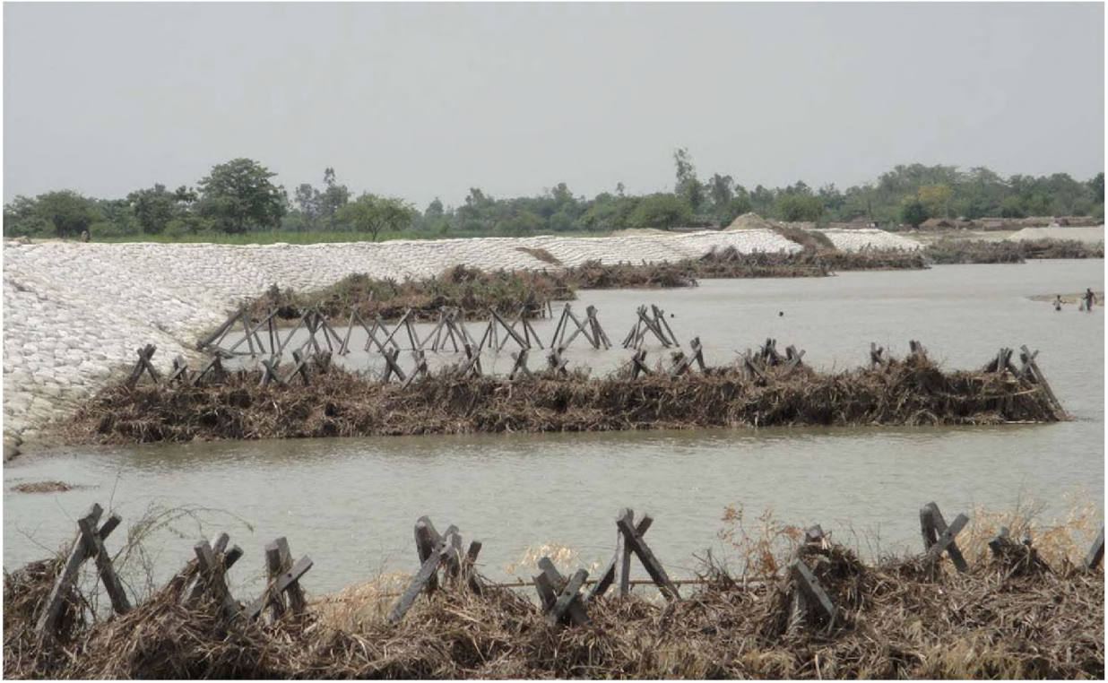
Geobag Pitching & Launching Apron with Procupines filled with jhankar on right bank of river Sarada in Village Ratuli, Uttar Pradesh
